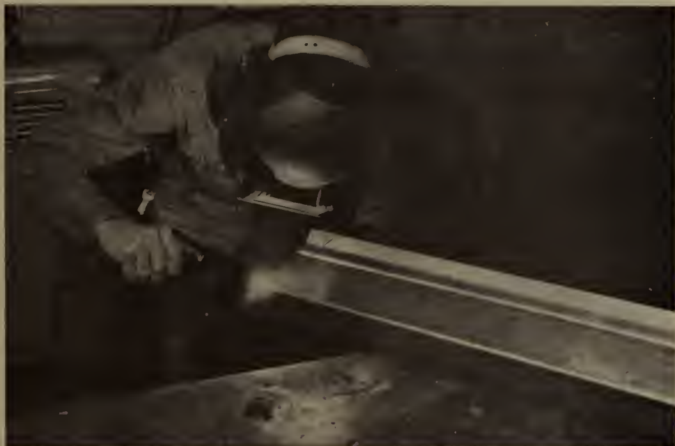
Welding a grill — Wayne Wilson, a craftsman whose primary job is welding, was named the Physical Plant's "Employee of the Year" for 1984. A fixer of everything from steam pipes to flush valves, Wilson here is welding a grill for the fire department.
